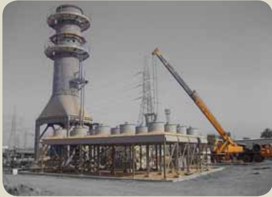
Taji Power Plant
